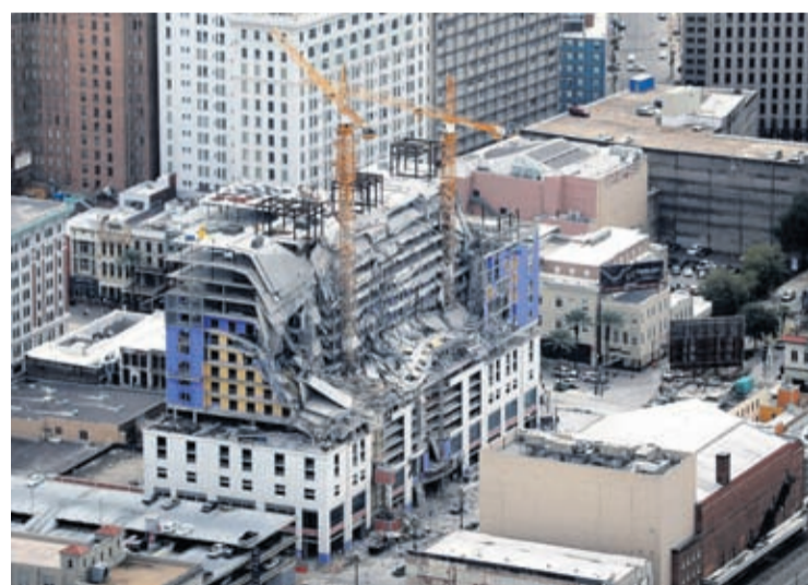
This Oct. 12, 2019, file photo shows damage of a partial collapse at the Hard Rock Hotel under construction in New Orleans.
